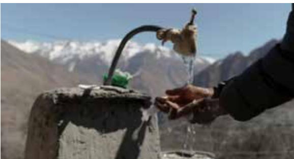
A tap wrapped in cloth (in Thuli Bheri, Dolpa/Nepal). This doesn't ensure water safety and highlights the important focus of water quality. Photo source: https://suswa.org/project/#what-we-do
