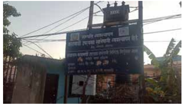
Local asset management: This information board near Sitapaila Chowk, Kathmandu, showcases the Kathmandu Valley Water Supply Management Board and its collaboration with Kathmandu Upatyaka Khanepati Limited to manage the Bahity Pump Station.
